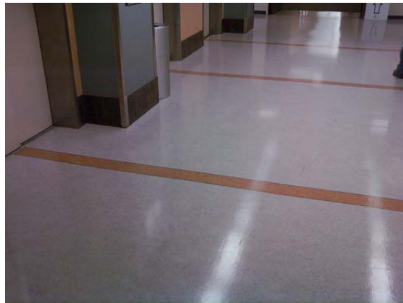
EPIC (predecessor) – after 2 years, linoleum in elevator area of large hospital
